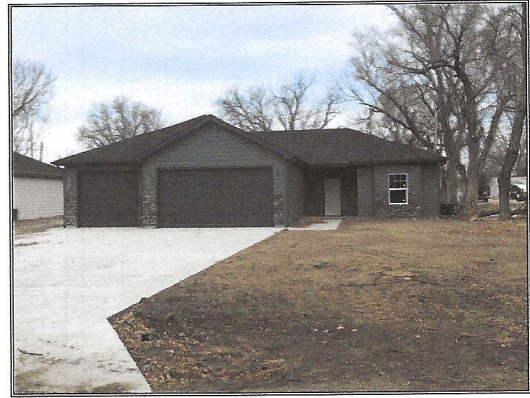
508 W. Sixth, Solomon, Kansas 3 bedroom, 2 bath, 3-car attached garage on slab under construction There were originally 3 40-year old mobile homes on the property Anticipate a $27,500.00 loss
