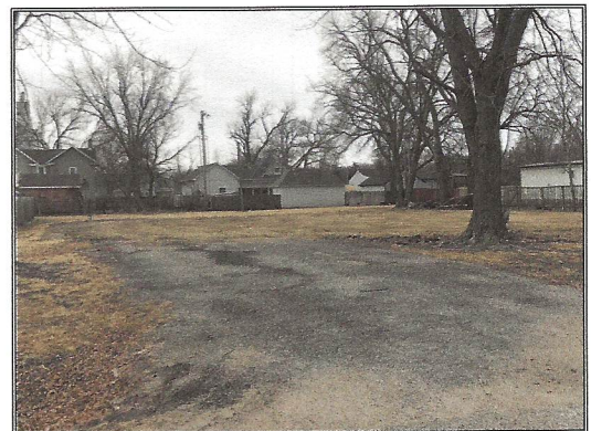
313 W. Sixth Street, Solomon, Kansas Mobile home removed, fill brought in to prepare for concrete pad. Intend to construct a 1,500 square foot, 3 bedroom, 2 bath, 3-car attached garage on slab. Anticipate a $30,000.00 loss
