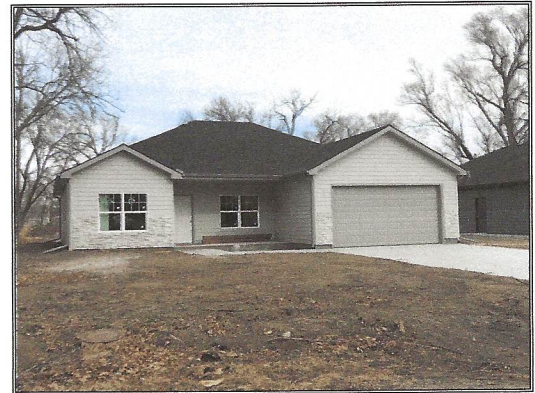
512 W. Sixth, Solomon, Kansas 3 bedroom, 2 bath, 2-car attached garage on slab under construction There were originally 3 40-year old mobile homes on the property Anticipate a $25,000.00 loss
