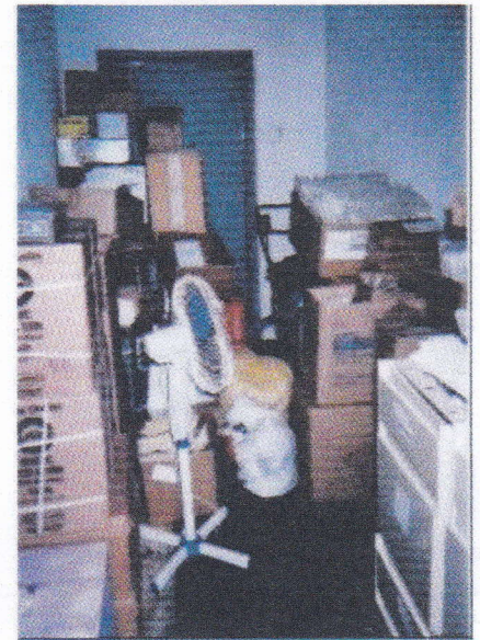
Fire hazard blocked back exit with lawn mower as a "back-up generator"
