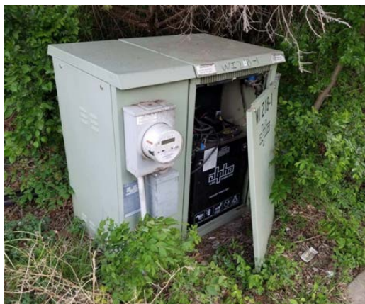
Power Supply After theft
