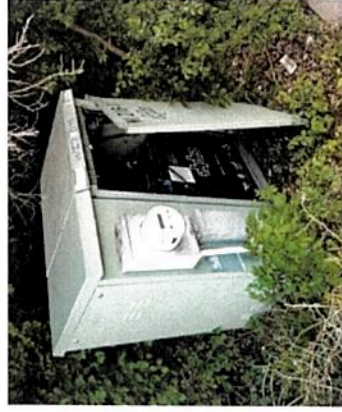
Power Supply After theft
