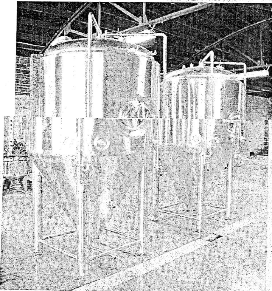
Two large tanks are some of the first pieces of brewing equipment set up in the brewery building. The operation will be fully visible from a large window on the sidewalk wall of the business.
