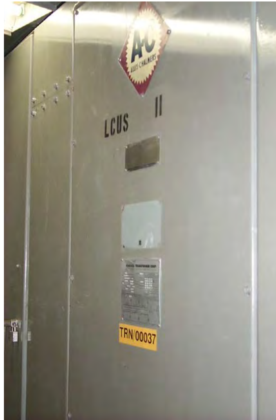
Picture #3528 Transformer LCUS-11 (TRN-00037) 300kva 13200V 208Y/120 7 th Floor-North Mech. Room
