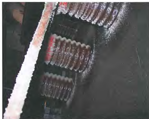
Photograph 2: 15 kV Copper Bus (Bottom view)
