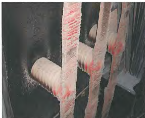
Photograph 1: 15 kV Vertical Copper Bus (Side view)
