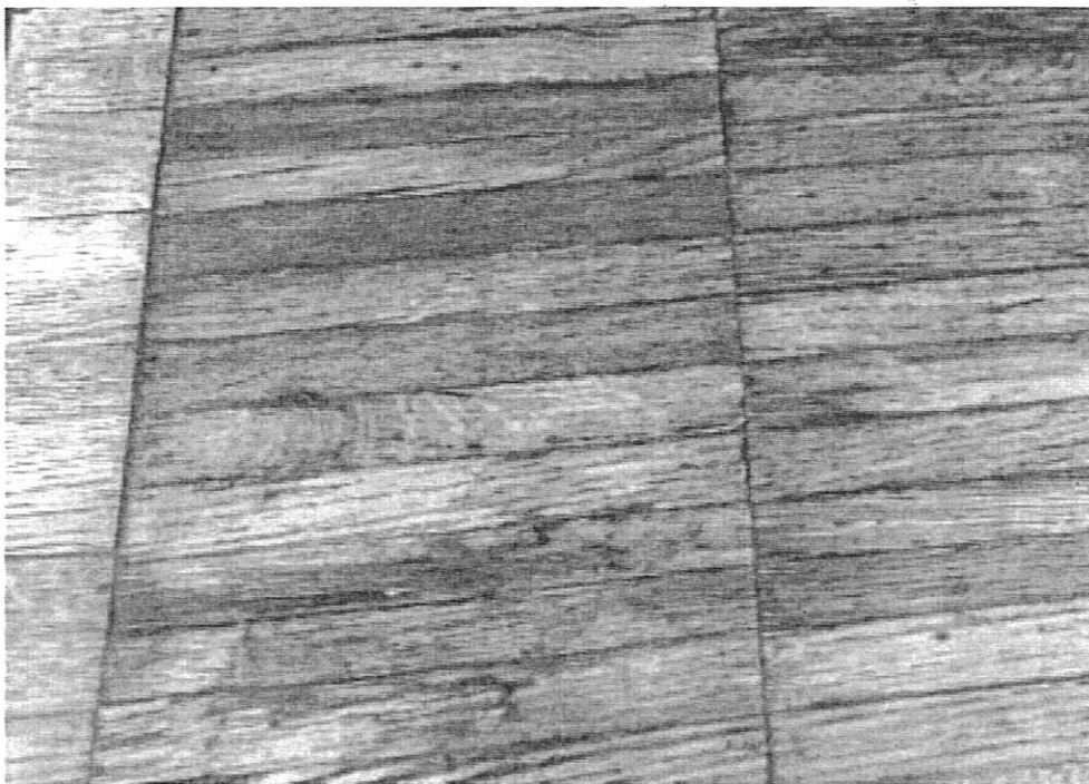
View of floor deterioration and patching
