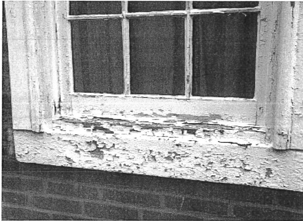
View of peeling paint
