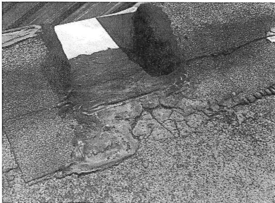
View of previous patching that is failing
