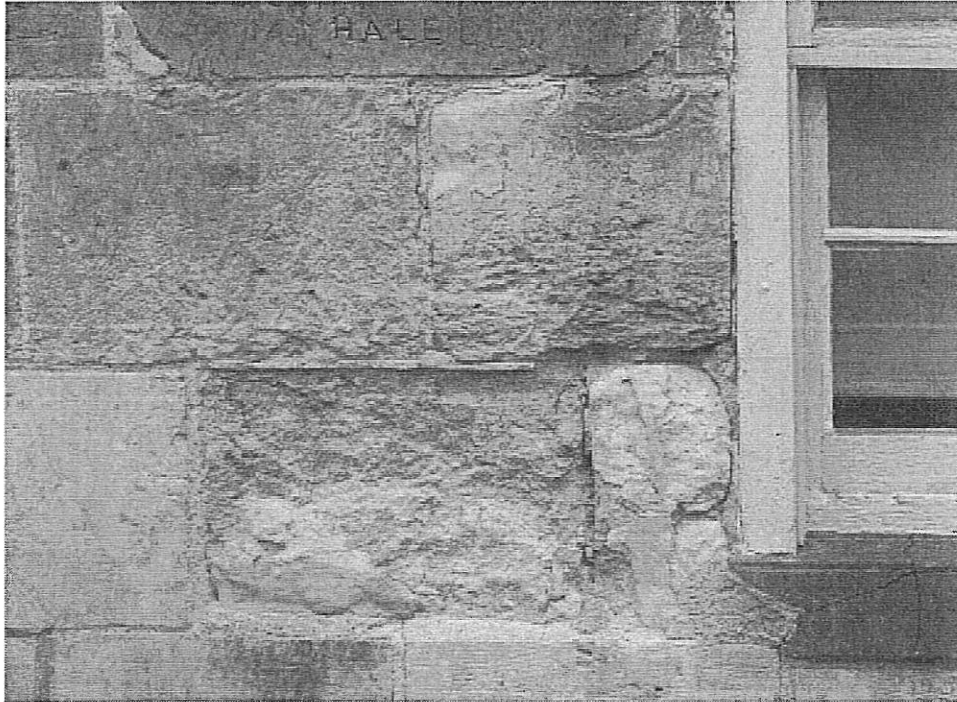
View of deteriorated and spalling stone
