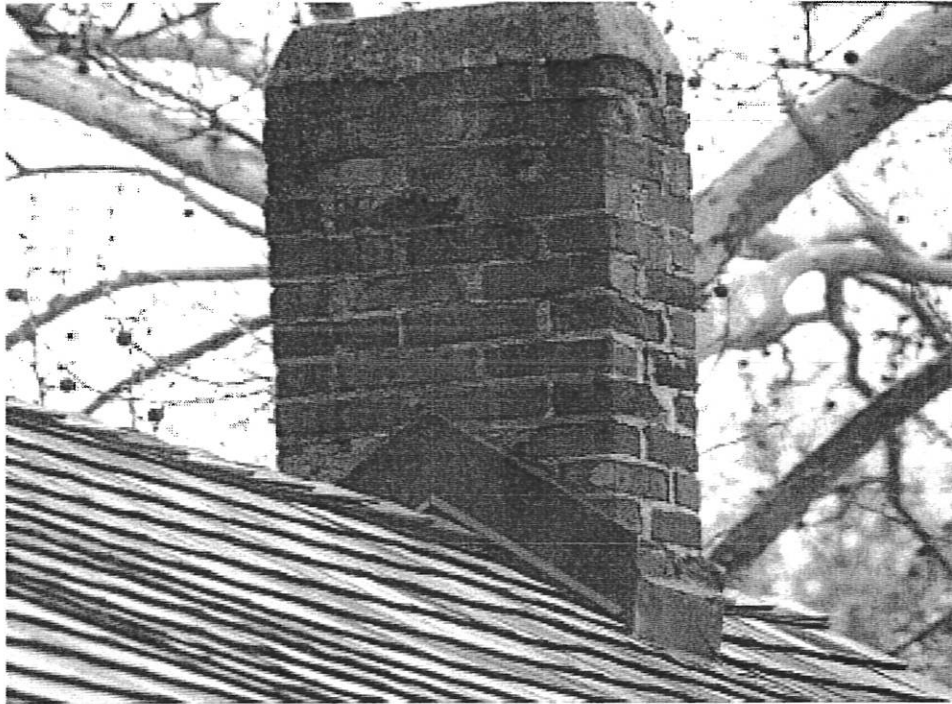
Brick chimney with damaged and spalling brick
