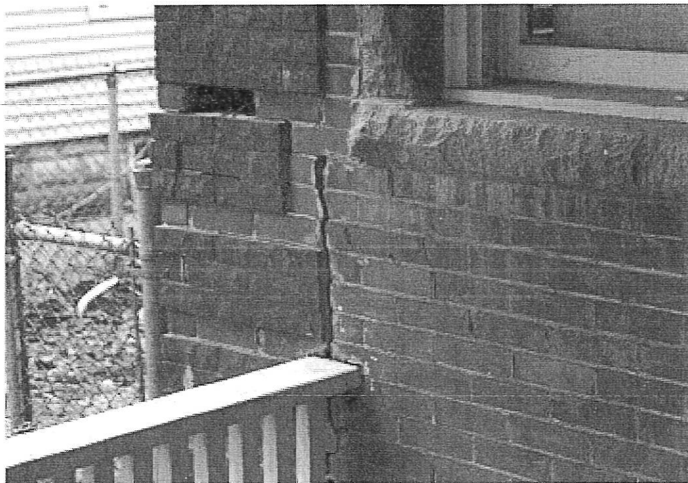
View showing missing brick and displaced corner
