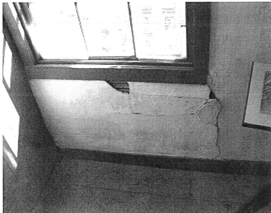
View of interior plaster damage
