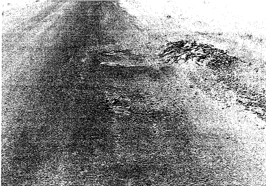
Figure 3 Rutting and potholes caused by trucks.
