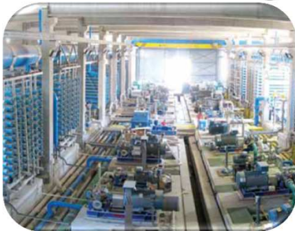
100.000 m 3 /day Desalination plant (India)
