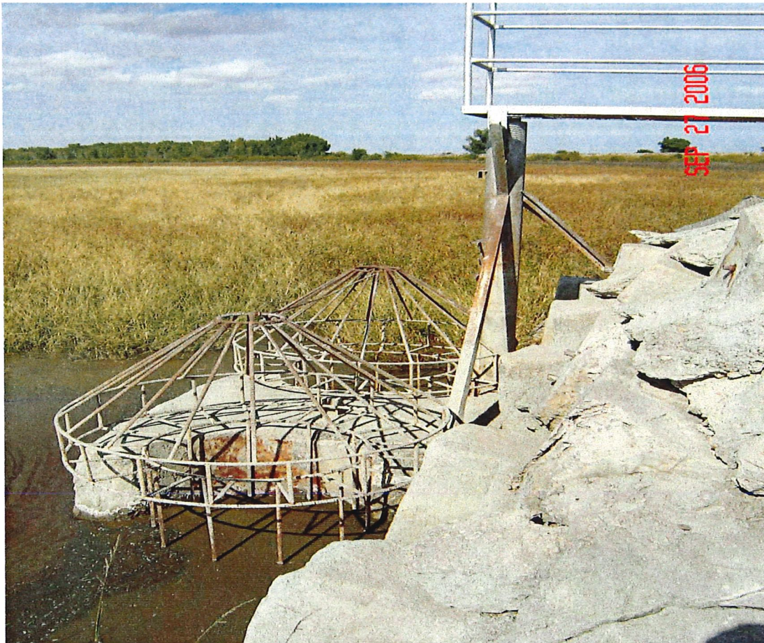
Old Outlet works with silt and grass indicating capacity loss in Lake McKinney
