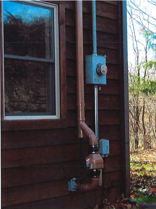
Exterior mounted radon fan
