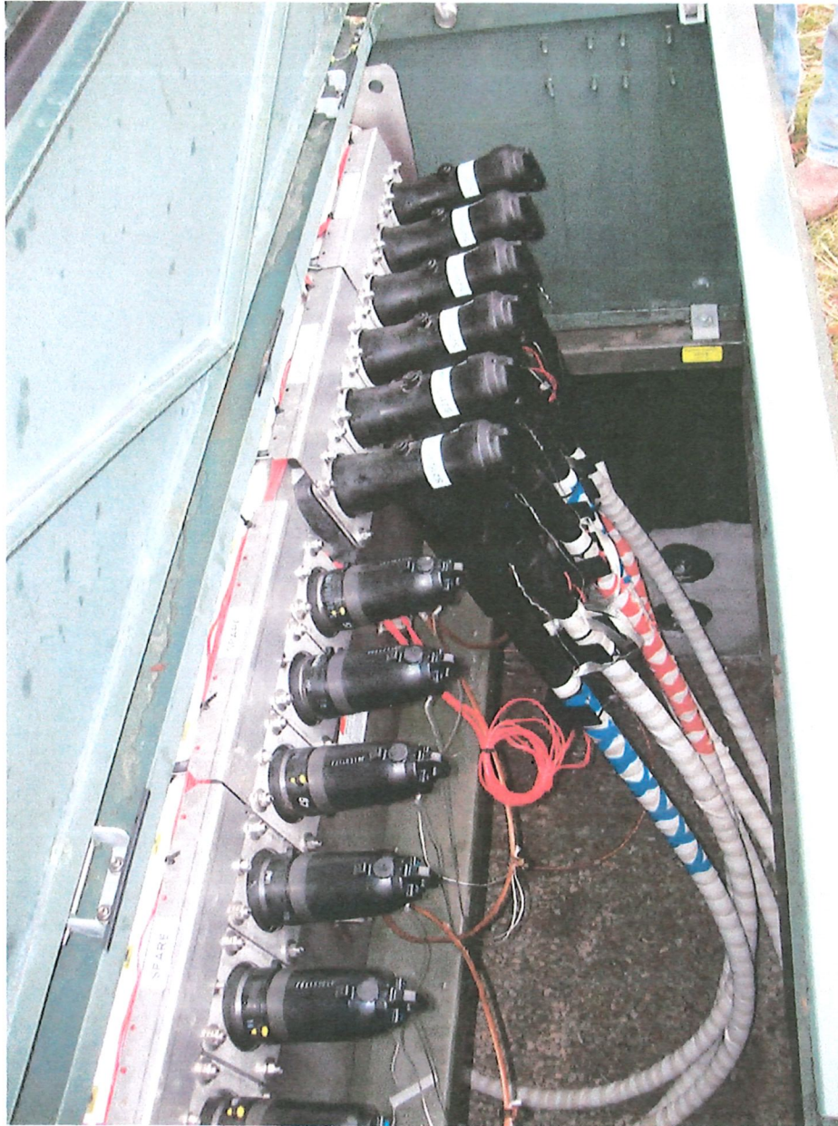
12.5 kV Switch Inputs From Electrical Substation
