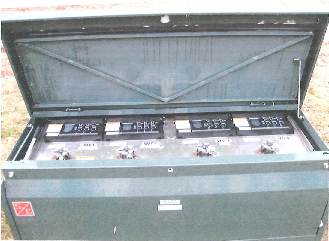
12.5 kV Switch Output Panels to Buildings
