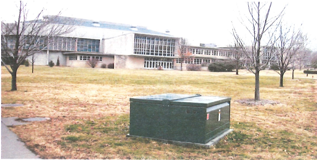
One 12.5 kV Switch Located Near Weber Hall
