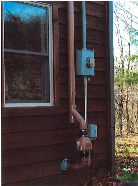
Exterior mounted radon fan
