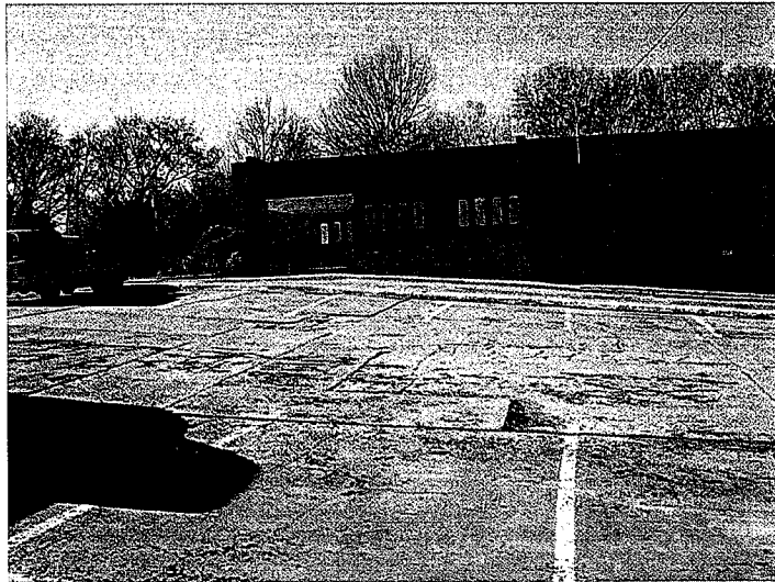
Crumbling Asphalt in Earl Center Parking Lot
