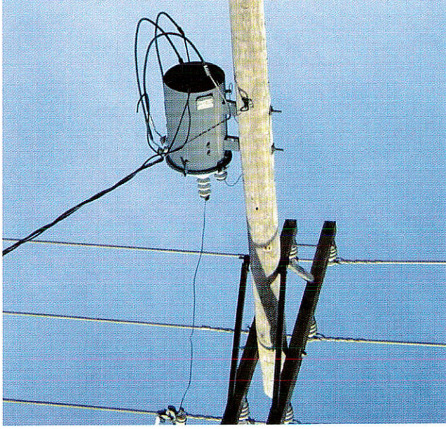
Above: A typical transformer in an older neighborhood that reduces electricity to 120 volts so it may be used in homes and businesses. Note the 3 wires. Two contain 120 volts each and the third is a ground wire. In neighborhoods with underground utilities the transformer is in a box located on the ground.
