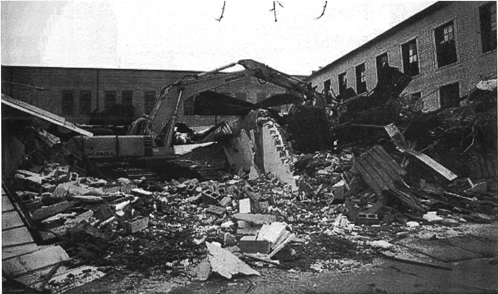
Demolition for construction of the new clinic/infirmarium in the maximum security unit at Lansing Correctional Facility.
