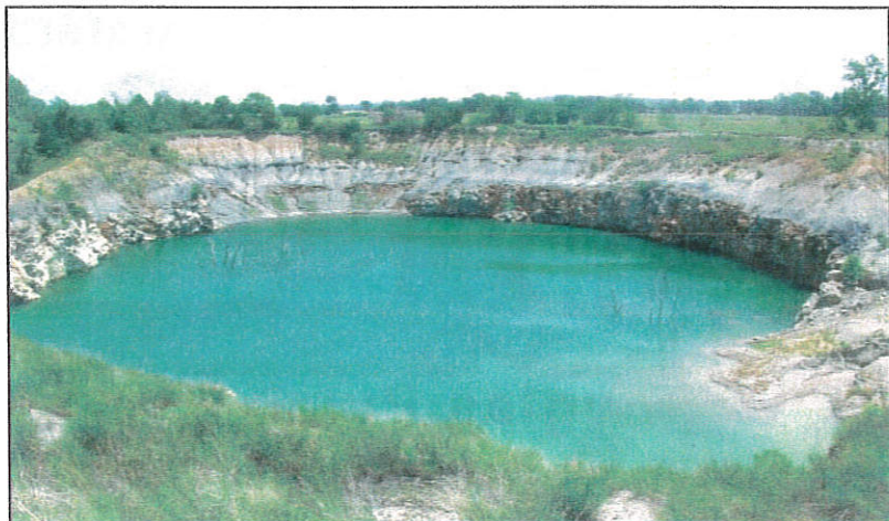
This image reflects what can happen to undermined areas where inadequate support is left in place. The cities of Treece, Kan. and Picher, Okla. are both in danger of experiencing subsidence such as this in residential areas of the communities.
