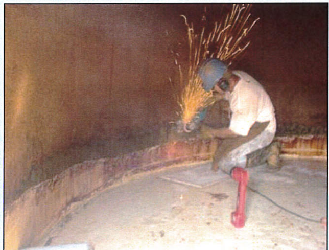
A Kansas Rural Water Association (KRWA) staff member repairs an emergency water leak in the City of Matfield Green's storage tank.
