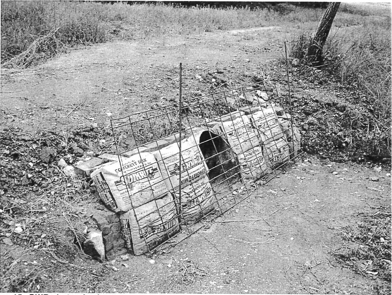
Figure 15. DWR photo of culvert gage constructed summer of 2005.
