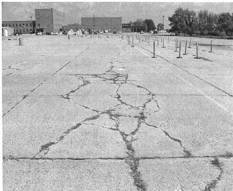
KLETC's concrete driving surface is deteriorating, exposing rebar
