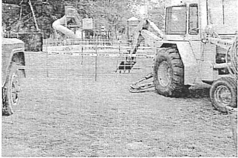
Abandoned Well in Schoolyard Lost Springs, KS
