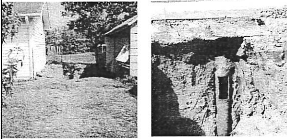
Abandoned Gas Well, Under House Foundation, Neodesha, KS
