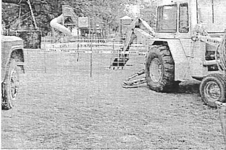
Abandoned Well in Schoolyard Lost Springs, KS
