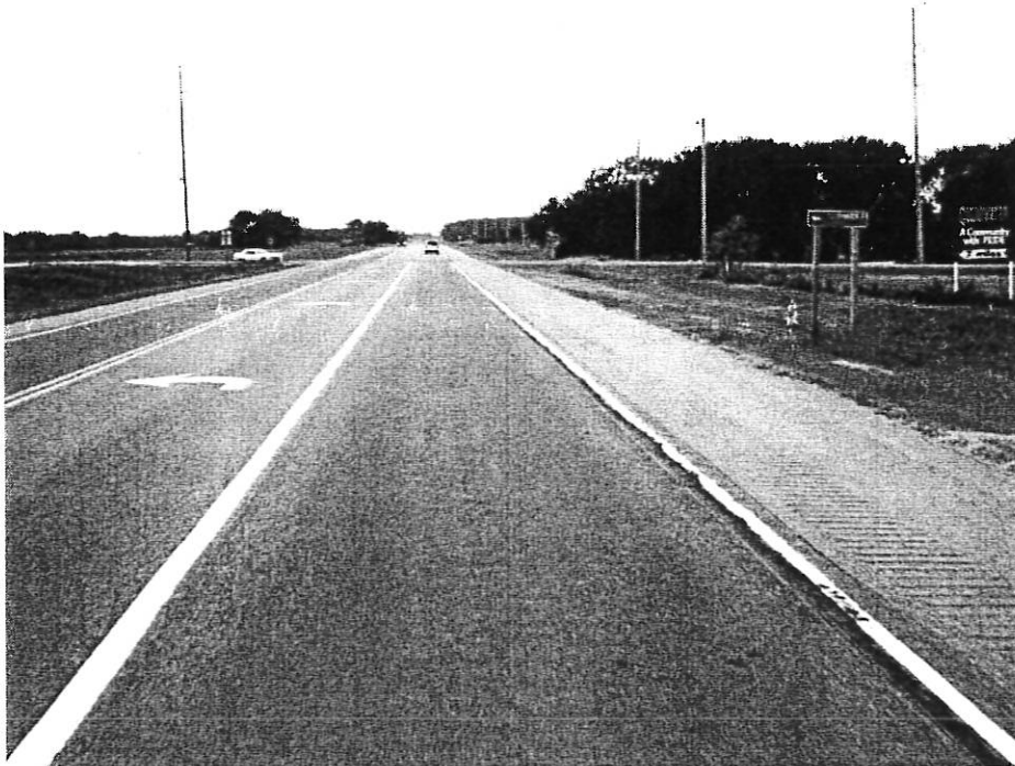
K-42, Westbound at a County Road "Clearwater 7, Left Arrow, Via County Road"
