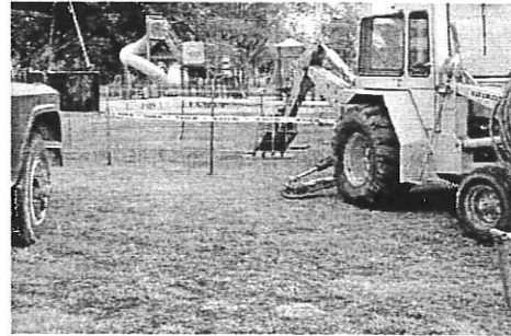
Abandoned Well in Schoolyard Lost Springs, KS
