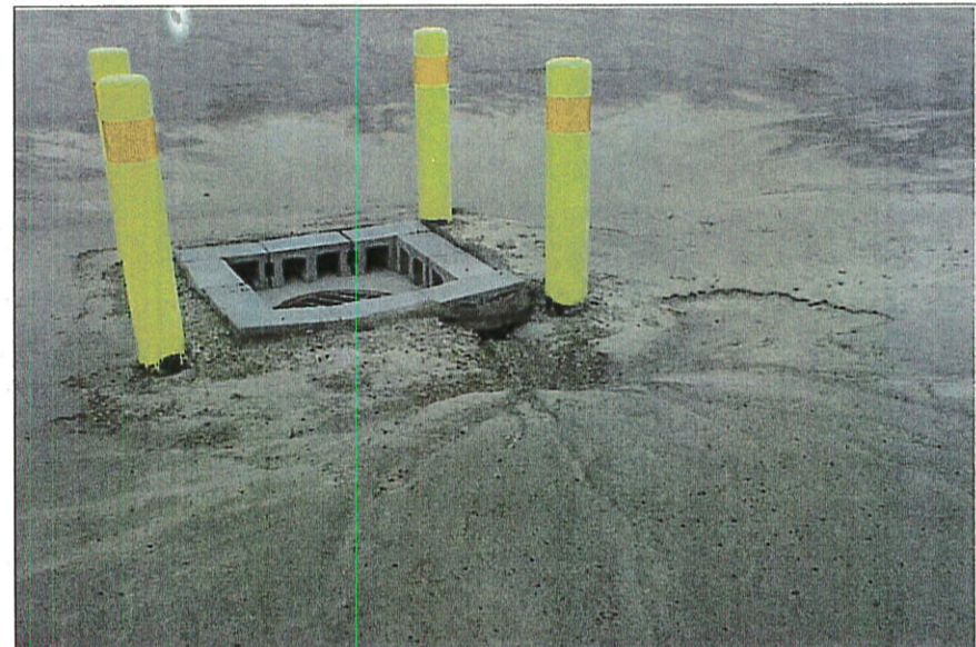
Erosion following completion
