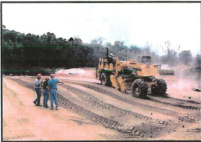
Stabilization of sludge waste. Impacted soils mixed with cement kiln dust to raise pH and demobilize subsurface waste.
