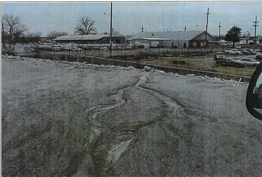
Erosion following completion
