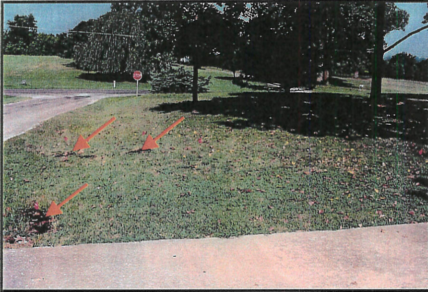
Residential property impacted by sludge mobilization and seepage.
