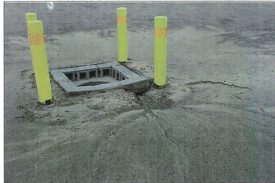
Erosion following completion
