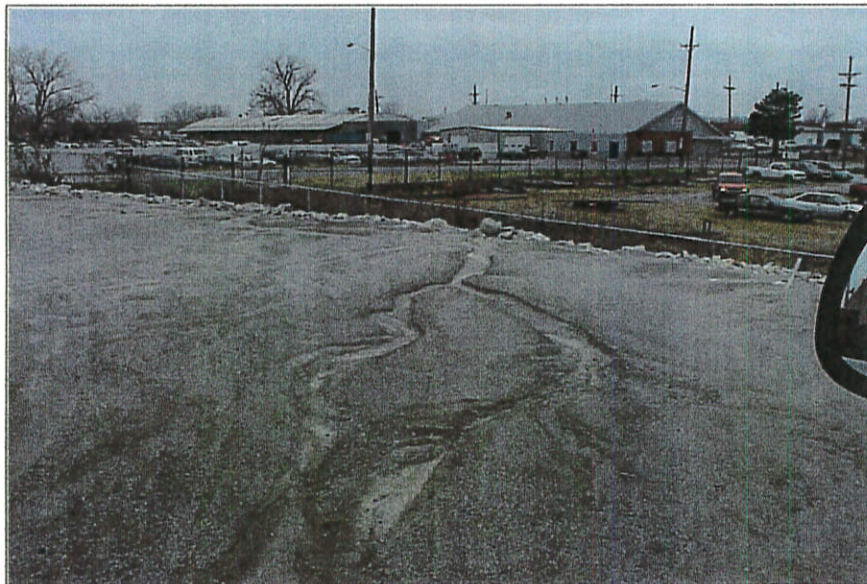
Erosion following completion
