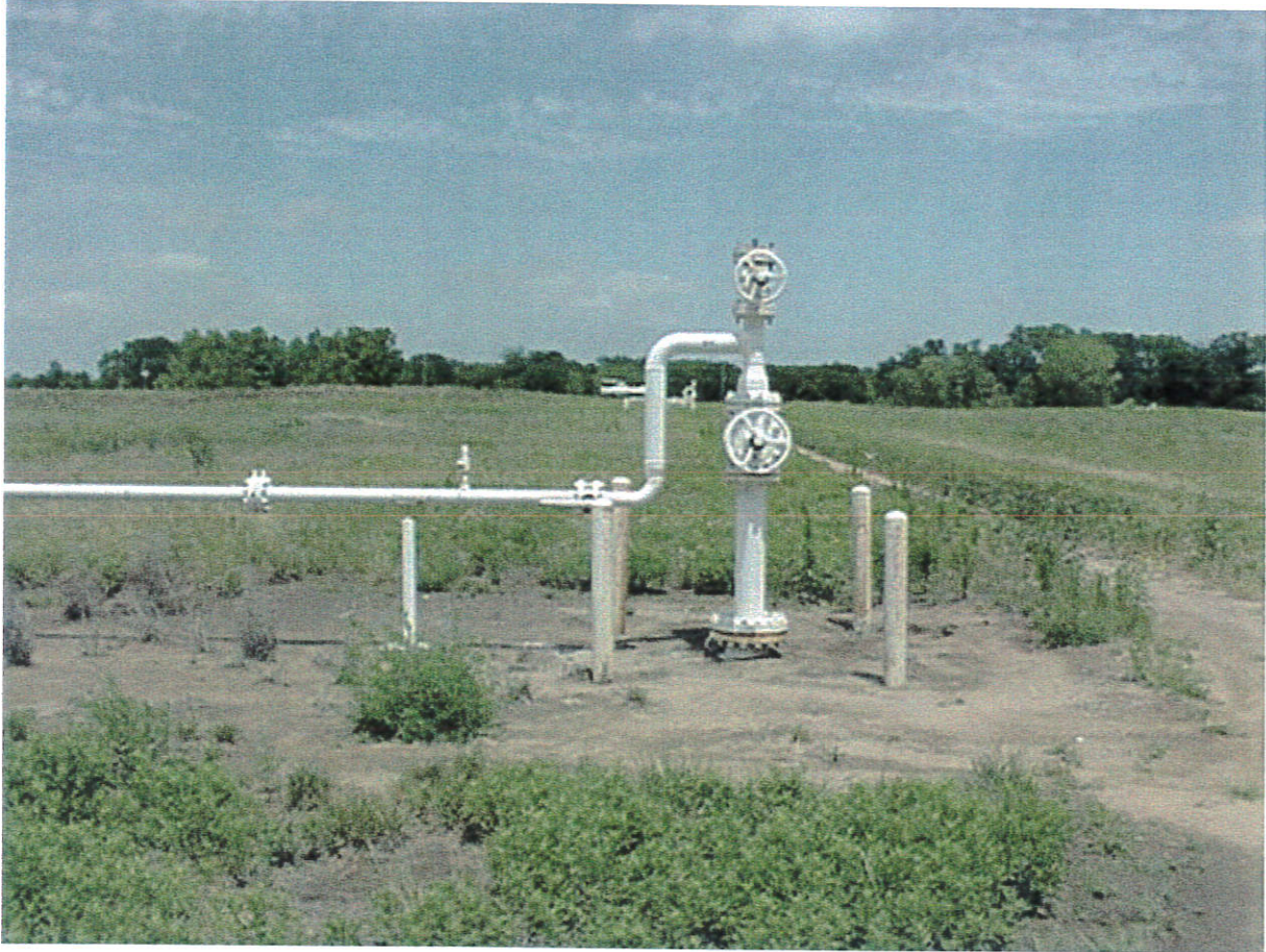
Kansas Gas Service Yaggy Facility Storage Well S-1
