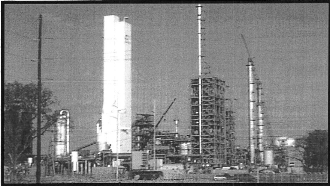
Nitrogen Fertilizer Facility
