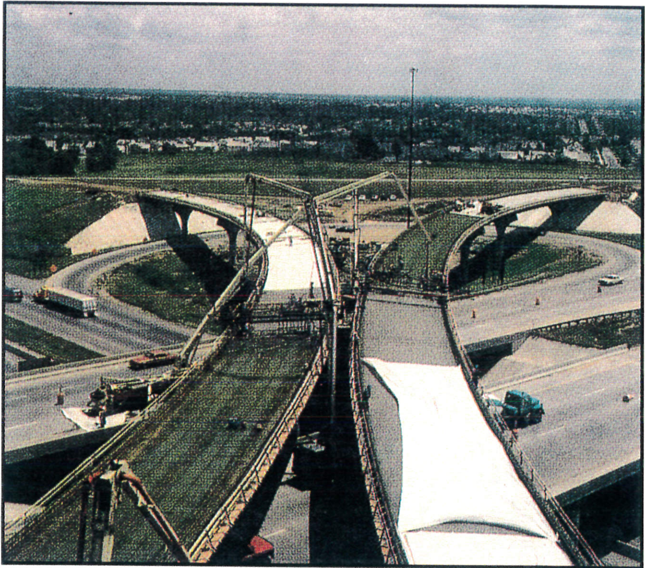
I-35 and I-435 Intersection, Overland Park, KS, 800 yard dual bridge placement using three KVM42 and one KVM36 138 ft. and 118 ft. boom trucks.
