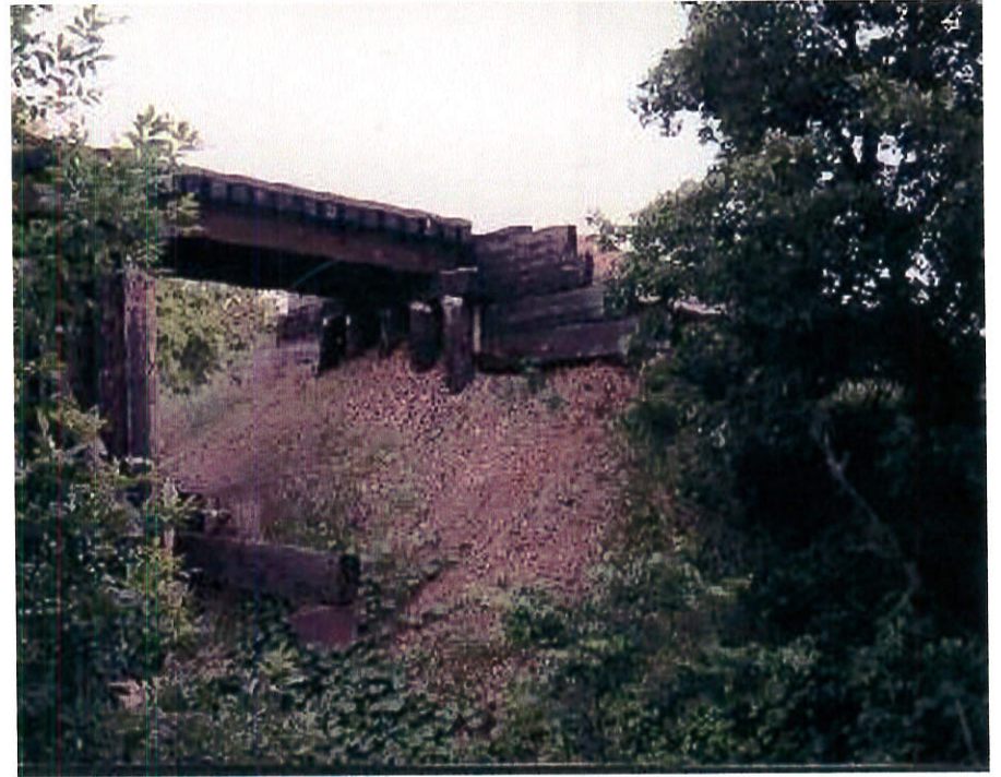
Bridge Unsuitable for Public Pedestrian Traffic
