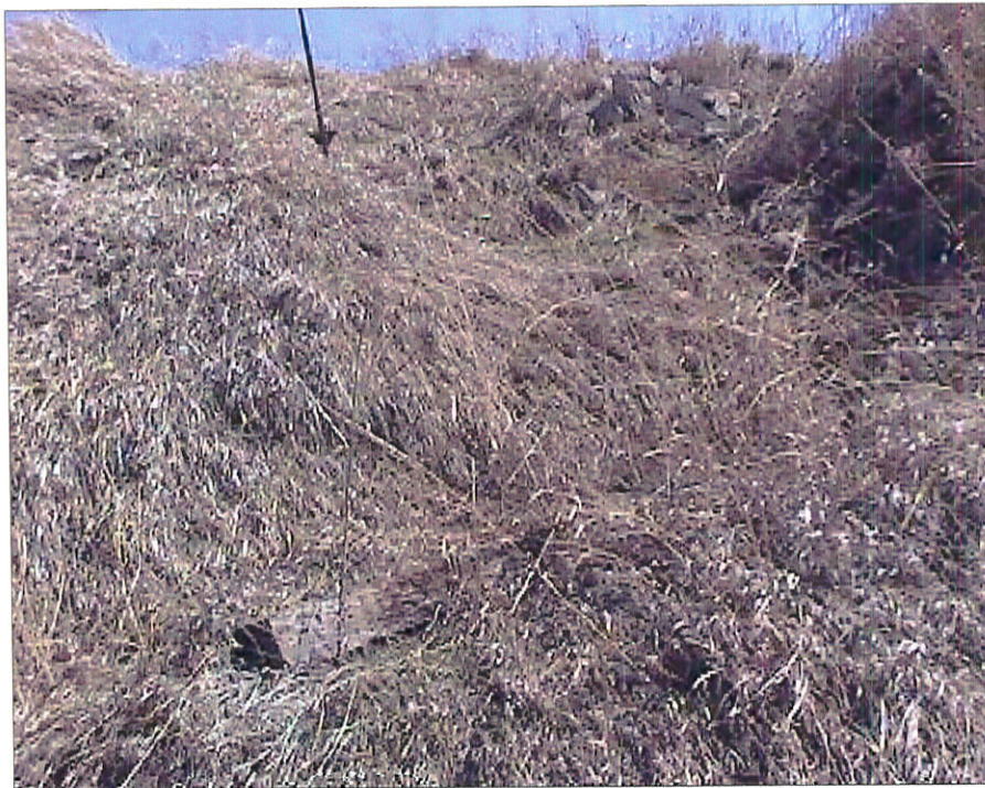
Erosion and / Abandoned Railroad Ties
