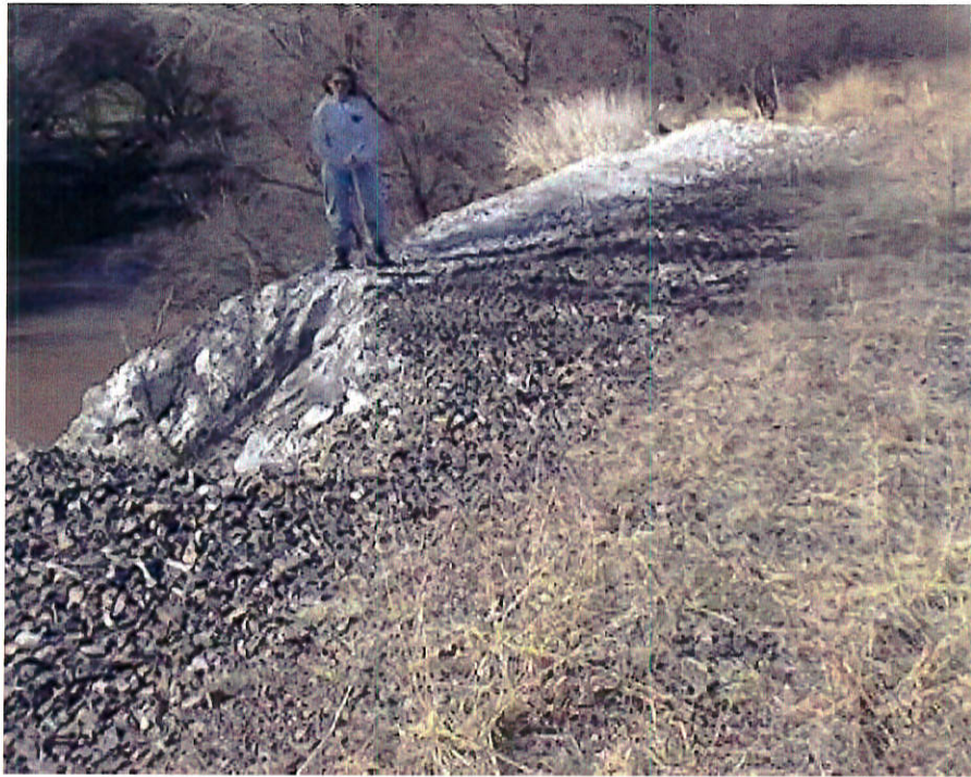
Erosion / 1/4 of Railroad Bed Gone
