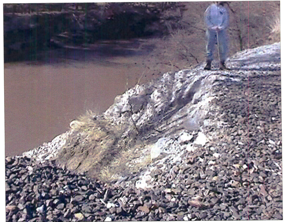
Erosion next to Smoky Hill River
