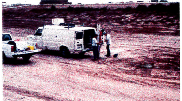
Right: Collecting soil cores from an 11-year-old lagoon using a direct-push soil probe. The lagoon had been dried and sludge removed prior to sampling.
