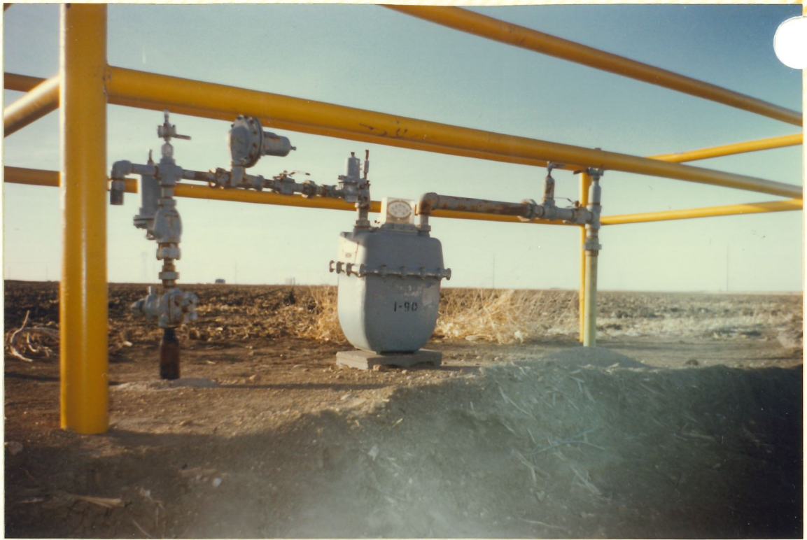
Example of equipment found at a typical irrigation "tap" on either the gathering system in the Hugoton Field, or a high pressure interstate pipeline transporting natural gas from the Field.
