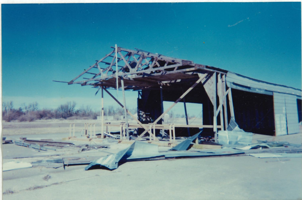
SHOWN: Loss of 1/4 of Aircraft Hanger Building Due to Tornado in Late 1995
