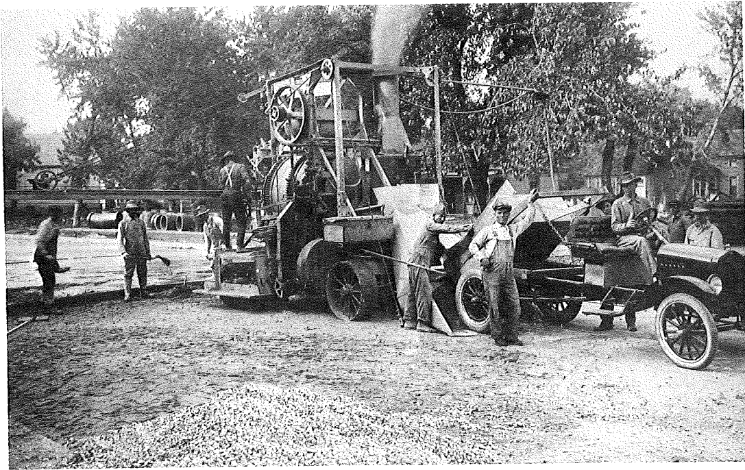
A paving mixer pulled by automobile pours concrete in Junction City in 1919.
