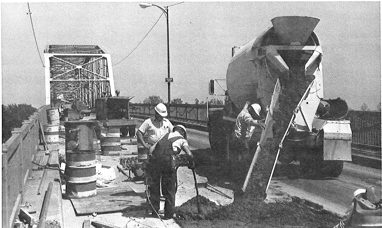
Reconstruction, rehabilitation and repair became the watchwords as KDOT worked to preserve the state's highway investment in the 1970s and 1980s.
