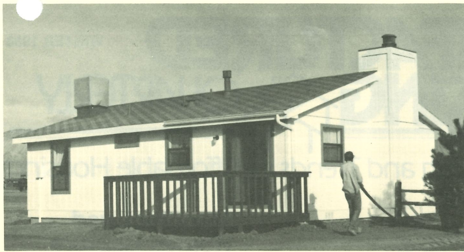
Typical multi-section manufactured home being installed in the Brookwood subdivision of Grand Junction, Colorado.
