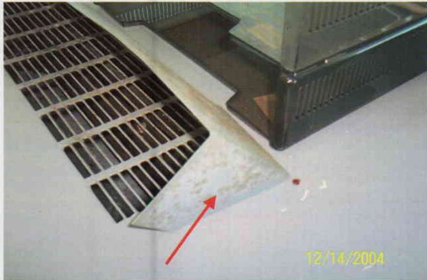
Photo No. 13 View of diffuser on 4 th floor ventilator. Note discoloration on diffuser. Arrow denotes location of sample T-10.
