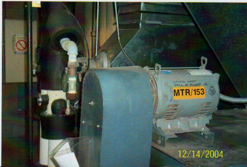
Photo No. 8 View of air handling unit in 4 th floor mechanical room.
