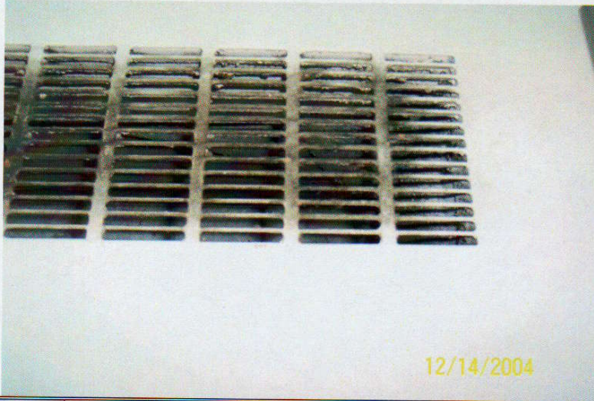
Photo No. 17 View of diffuser on 4 th floor ventilator. Note discoloration on diffuser.
