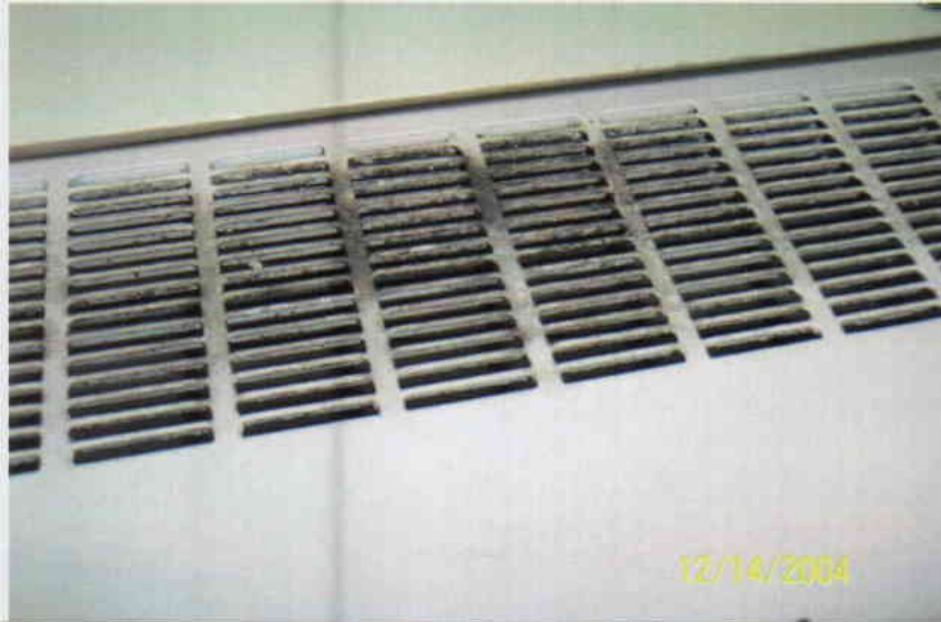
Photo No. 15 View of diffuser on 4 th floor ventilator. Note discoloration on diffuser.
