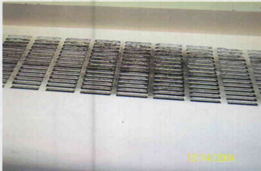
Photo No. 14 View of diffuser on 4 th floor ventilator. Note discoloration on diffuser.
