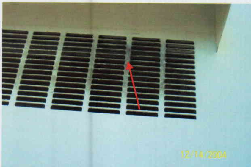
Photo No. 4 View of diffuser on 10 th floor ventilator. Note discoloration on diffuser. Arrow denotes location of sample T-11.
