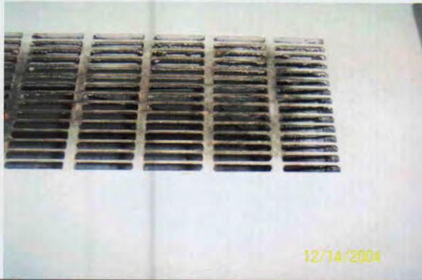
Photo No. 17 View of diffuser on 4 th floor ventilator. Note discoloration on diffuser.
