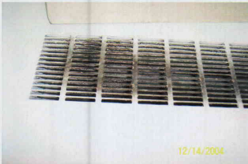
Photo No. 16 View of diffuser on 4 th floor ventilator. Note discoloration on diffuser.
