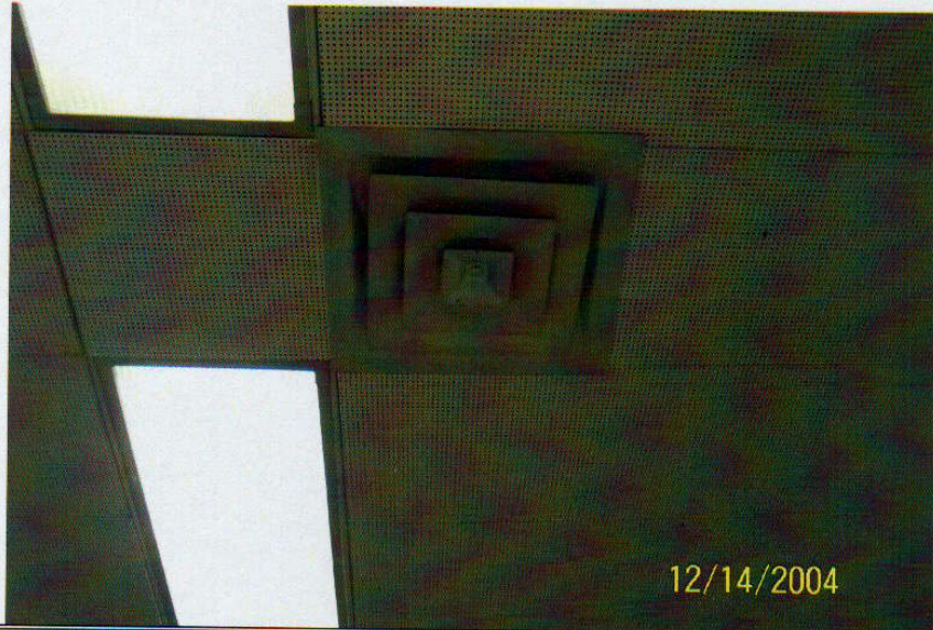
Photo No. 3 View of ceiling air diffuser located on 10 th floor. Diffuser appears to be relatively clean with no evidence of fungal growth. Typical of all diffusers on 10 th floor.
