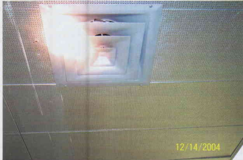
Photo No. 11 View of ceiling air diffuser located on 4 th floor. Diffuser appears to be relatively clean with no evidence of fungal growth. Typical of all diffusers on 4 th floor.
