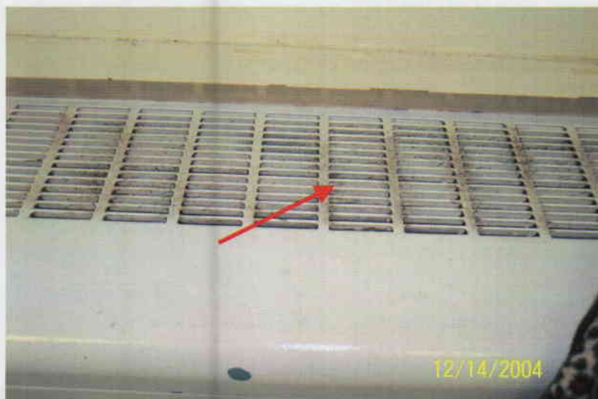
Photo No. 7 View of diffuser on 10 th floor ventilator. Note discoloration on diffuser. Arrow denotes location of sample T-13.
