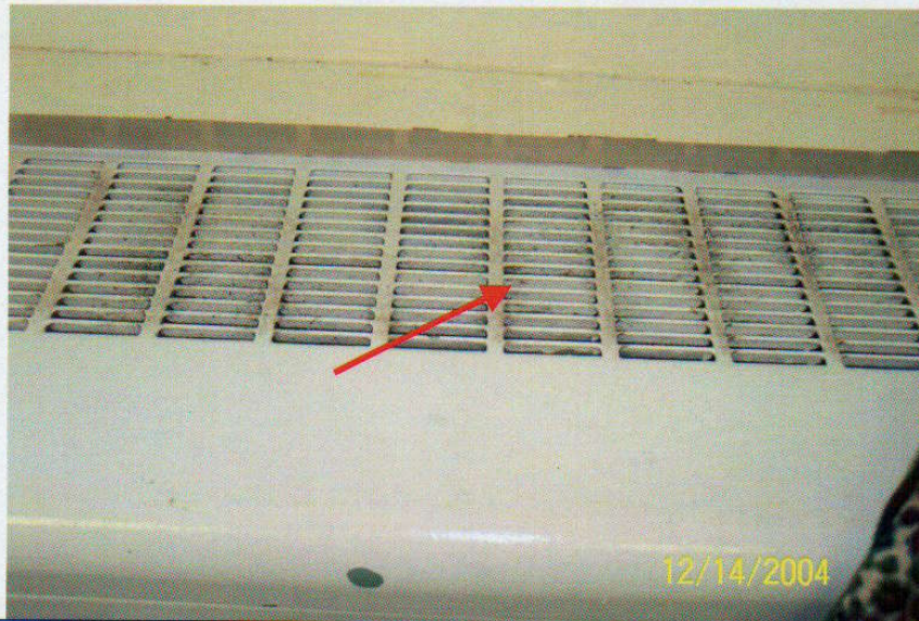
Photo No. 7 View of diffuser on 10 th floor ventilator. Note discoloration on diffuser. Arrow denotes location of sample T-13.
