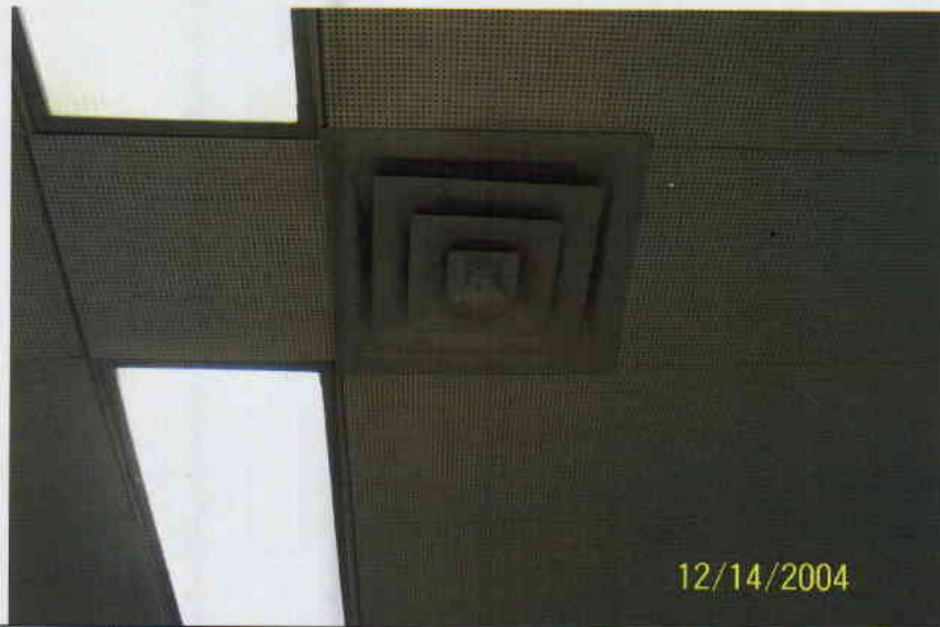
Photo No. 3 View of ceiling air diffuser located on 10 th floor. Diffuser appears to be relatively clean with no evidence of fungal growth. Typical of all diffusers on 10 th floor.
