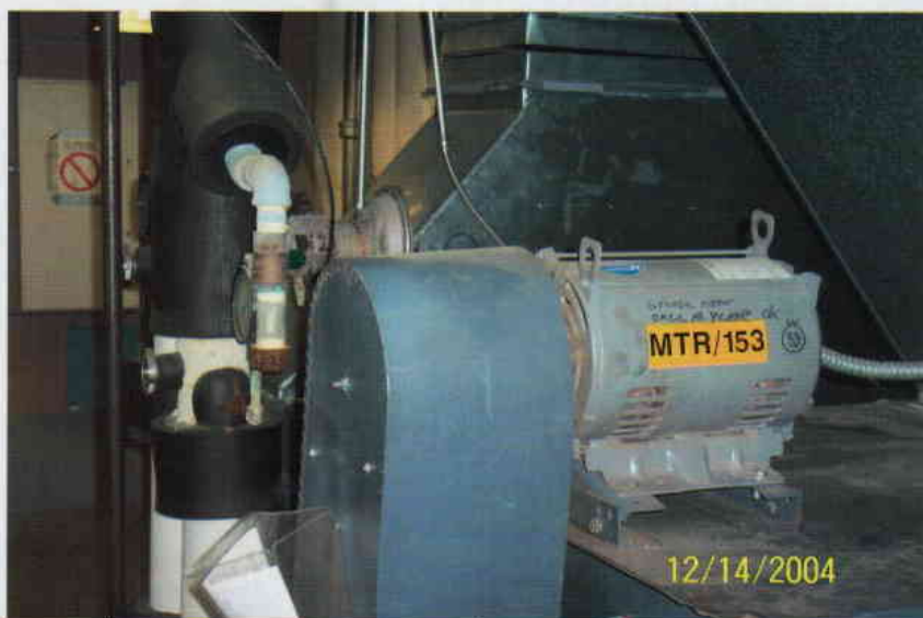
Photo No. 8 View of air handling unit in 4 th floor mechanical room.
