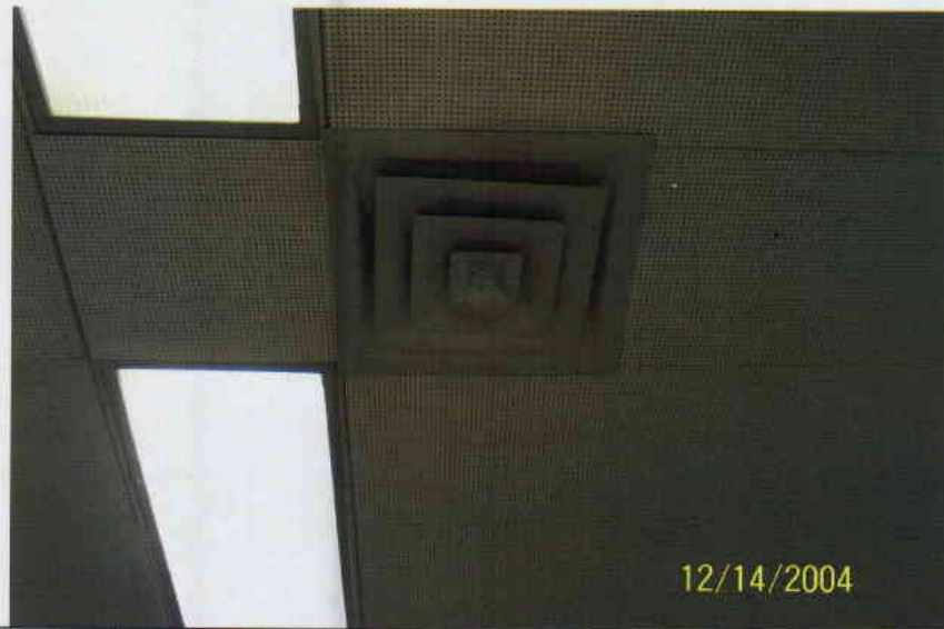
Photo No. 3 View of ceiling air diffuser located on 10 th floor. Diffuser appears to be relatively clean with no evidence of fungal growth. Typical of all diffusers on 10 th floor.
