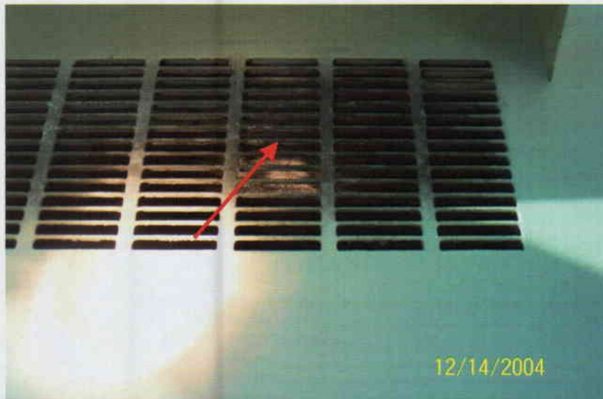
Photo No. 10 View of diffuser on 4 th floor ventilator. Note discoloration on diffuser. Arrow denotes location of sample T-08.
