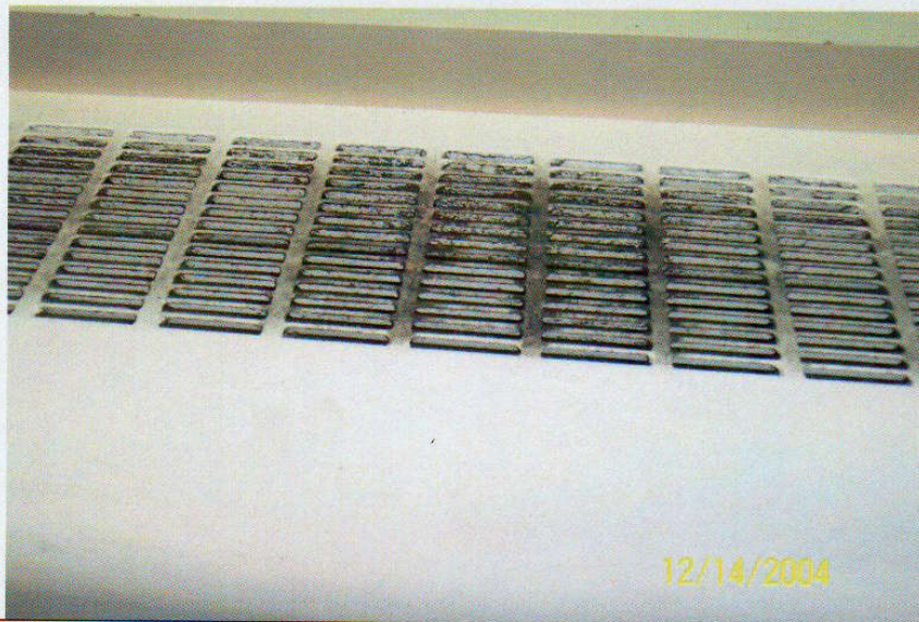
Photo No. 14 View of diffuser on 4 th floor ventilator. Note discoloration on diffuser.
