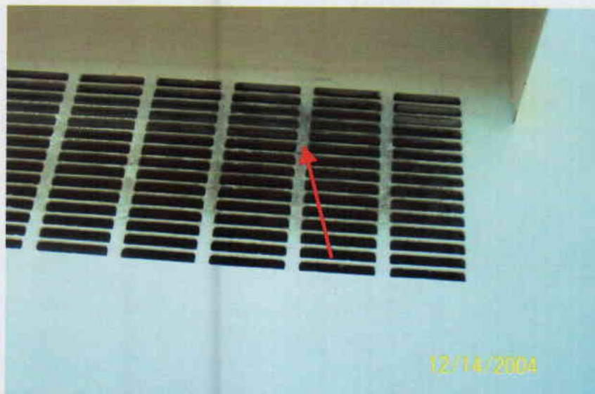
Photo No. 4 View of diffuser on 10 th floor ventilator. Note discoloration on diffuser. Arrow denotes location of sample T-11.
