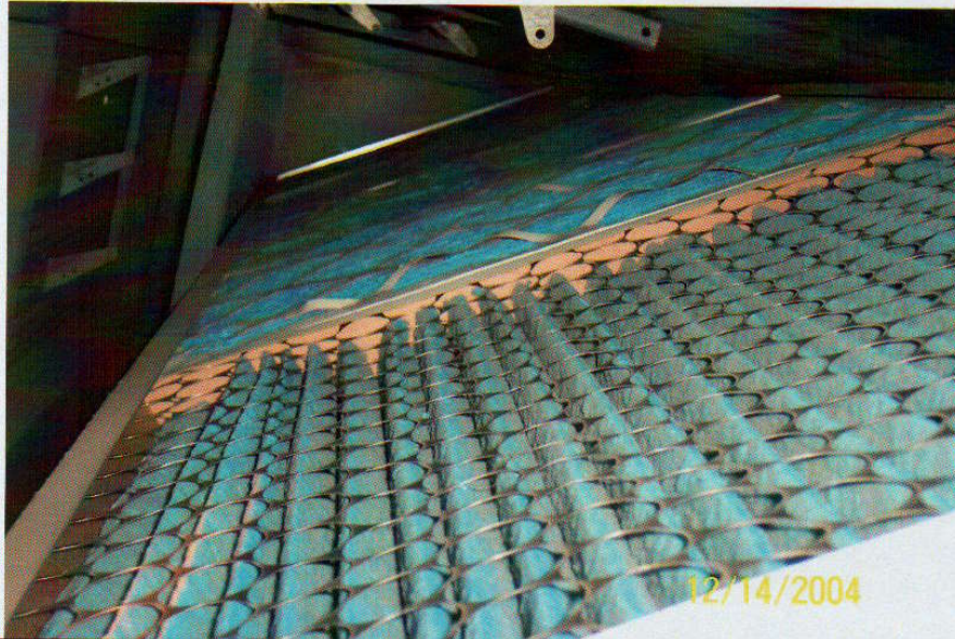
Photo No. 9 View of filters in 4 th floor air handling unit. Filters appear to be well maintained with no build-up of excessive dust or debris.
