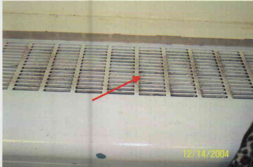
Photo No. 7 View of diffuser on 10 th floor ventilator. Note discoloration on diffuser. Arrow denotes location of sample T-13.
