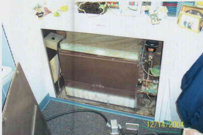
Photo No. 5 View inside 10 th floor ventilator unit.
