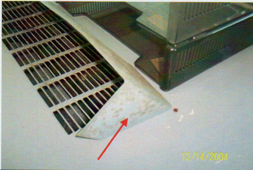
Photo No. 13 View of diffuser on 4 th floor ventilator. Note discoloration on diffuser. Arrow denotes location of sample T-10.
