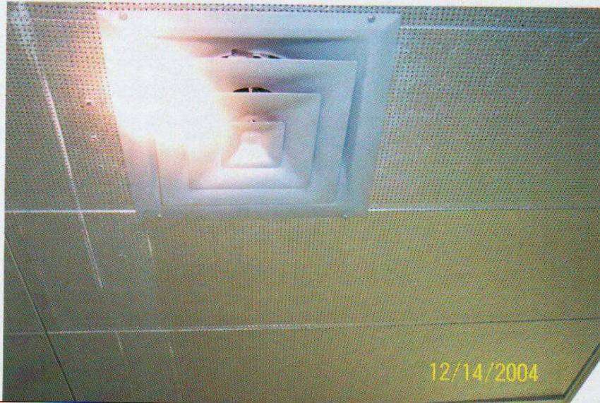
Photo No. 11 View of ceiling air diffuser located on 4 th floor. Diffuser appears to be relatively clean with no evidence of fungal growth. Typical of all diffusers on 4 th floor.
