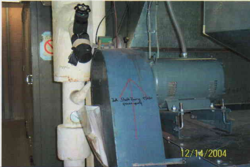
Photo No. 1 View of air handling unit in 10 th floor mechanical room.
