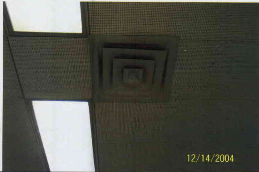
Photo No. 3 View of ceiling air diffuser located on 10 th floor. Diffuser appears to be relatively clean with no evidence of fungal growth. Typical of all diffusers on 10 th floor.
