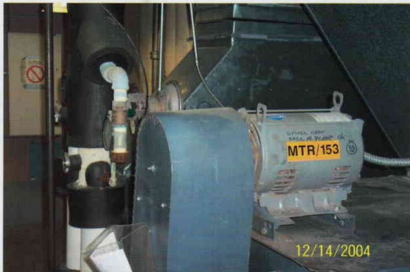
Photo No. 8 View of air handling unit in 4 th floor mechanical room.
