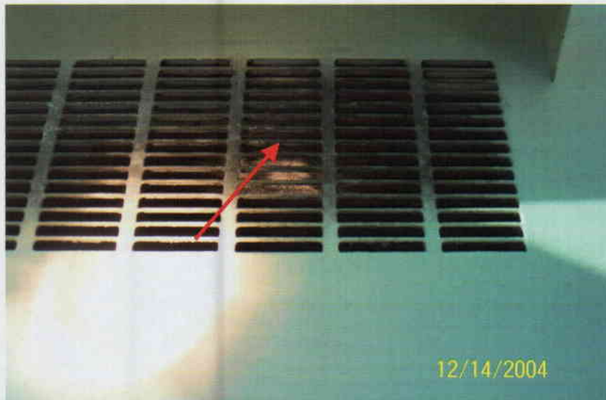
Photo No. 10 View of diffuser on 4 th floor ventilator. Note discoloration on diffuser. Arrow denotes location of sample T-08.
