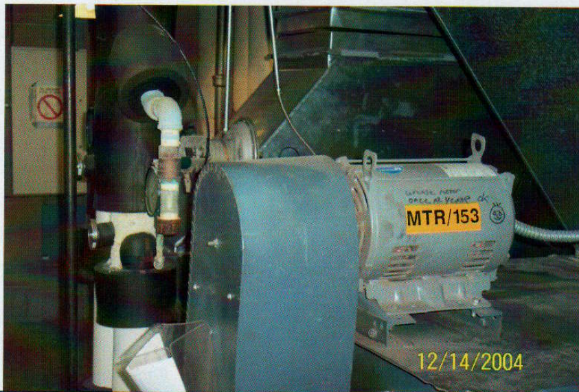
Photo No. 8 View of air handling unit in 4 th floor mechanical room.
