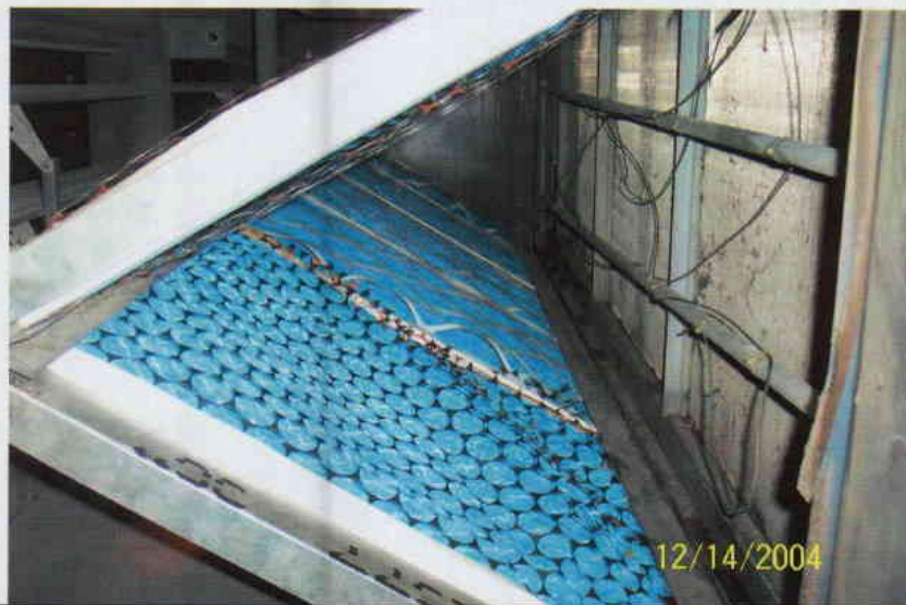
Photo No. 2 View of filters in 10 th floor air handling unit. Filters appear to be well maintained with no build-up of excessive dust or debris.
