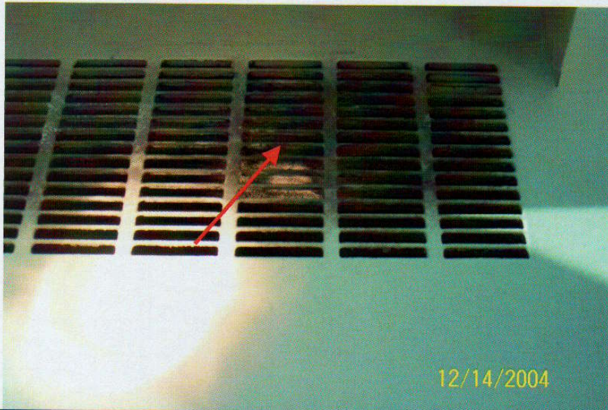
Photo No. 10 View of diffuser on 4 th floor ventilator. Note discoloration on diffuser. Arrow denotes location of sample T-08.
