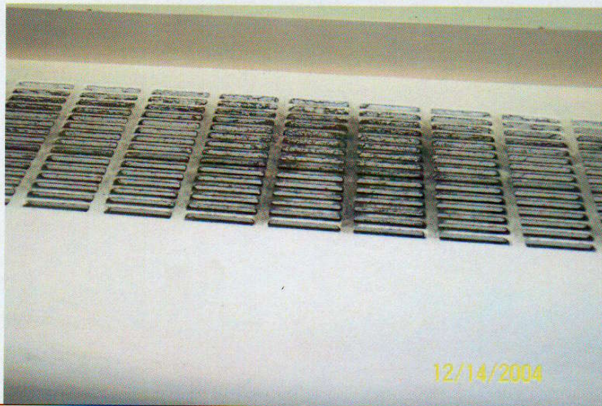
Photo No. 14 View of diffuser on 4 th floor ventilator. Note discoloration on diffuser.
