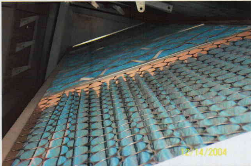
Photo No. 9 View of filters in 4 th floor air handling unit. Filters appear to be well maintained with no build-up of excessive dust or debris.
