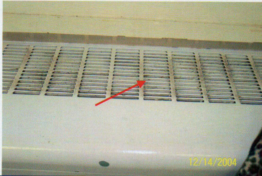
Photo No. 7 View of diffuser on 10 th floor ventilator. Note discoloration on diffuser. Arrow denotes location of sample T-13.
