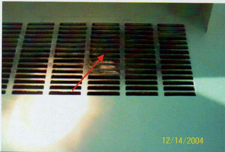
Photo No. 10 View of diffuser on 4 th floor ventilator. Note discoloration on diffuser. Arrow denotes location of sample T-08.
