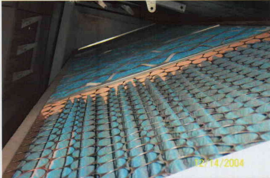
Photo No. 9 View of filters in 4 th floor air handling unit. Filters appear to be well maintained with no build-up of excessive dust or debris.
