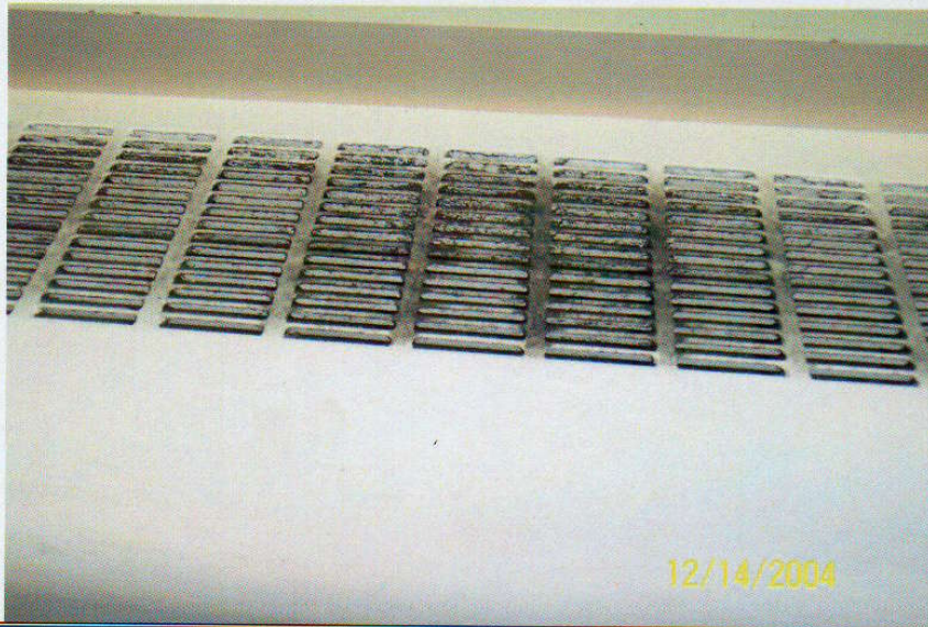
Photo No. 14 View of diffuser on 4 th floor ventilator. Note discoloration on diffuser.
